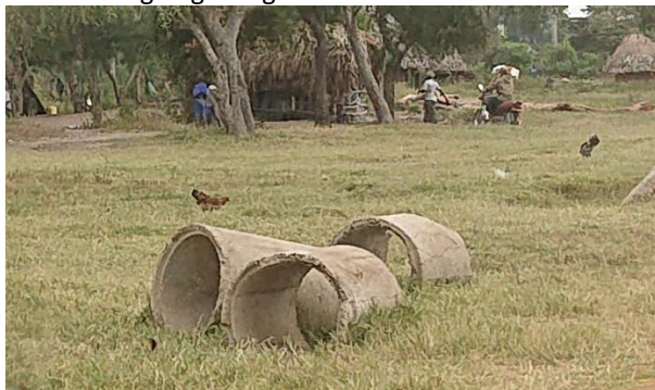
C: Damage of culverts
