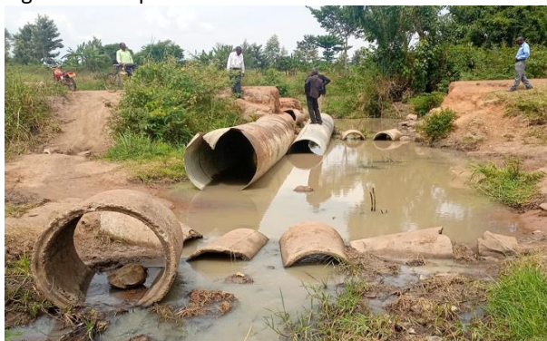
D: Damage of road infrastructure Budumba SC
