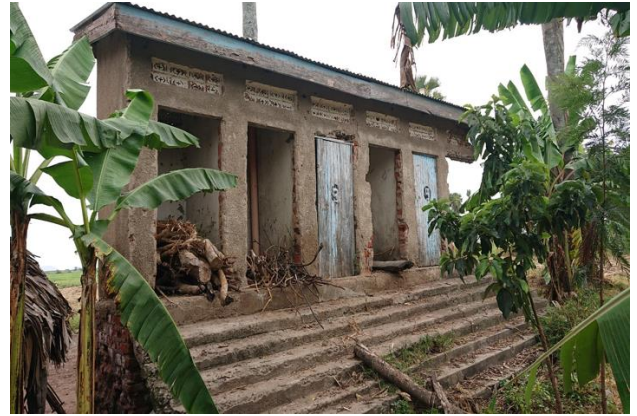
3.6. B: Destruction of WASH Facilities
